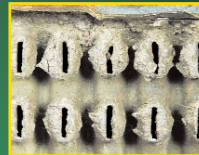
Rust, scale and sludge can plug cooling system fins, preventing proper circulation of coolant.
